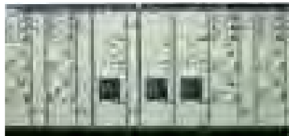
Withdrawable-type PCC and MCC
