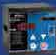
RX232 Power Fault Relay
