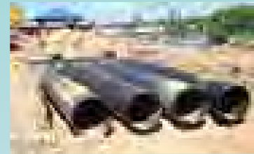
On-Site Stormwater Detention Tank at Balai Polis Bongawan, Kota Kinabalu, Sabah
