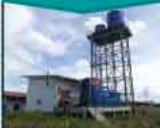
WATER FILTRATION SYSTEMS
