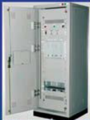
RTU for Power SCADA System
