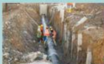
Drainage System at Mapai Substation, Kanowit
