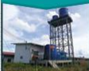
WATER FILTRATION SYSTEMS
